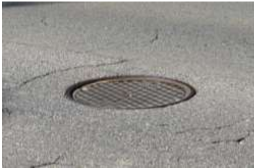
Sunken Plate at intersection w Ridge Ave
