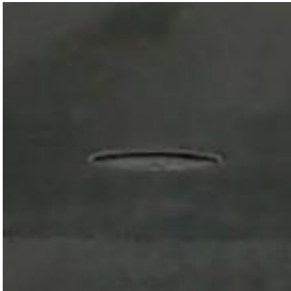
Sunken Plate at intersection w Montgomery Rd
