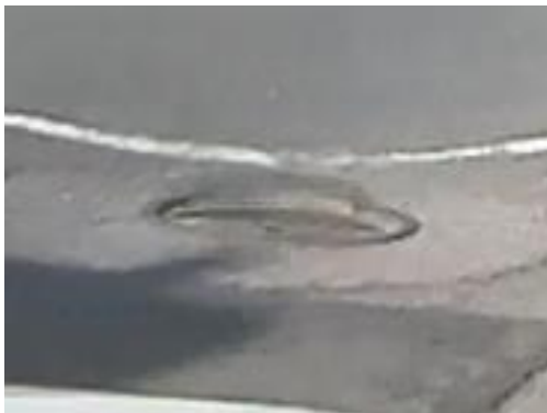
Sunken Plate at intersection w Spains Rd
