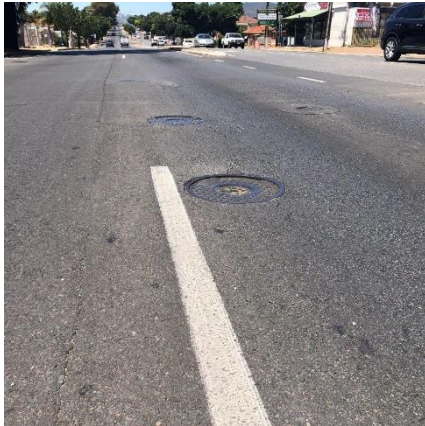
Sunken plate near Ashleigh St intersection w Payneham Rd
