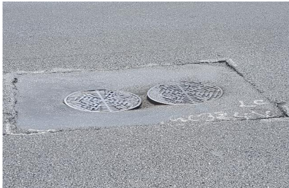
Pit covers at the intersection of Lorraine Ave
