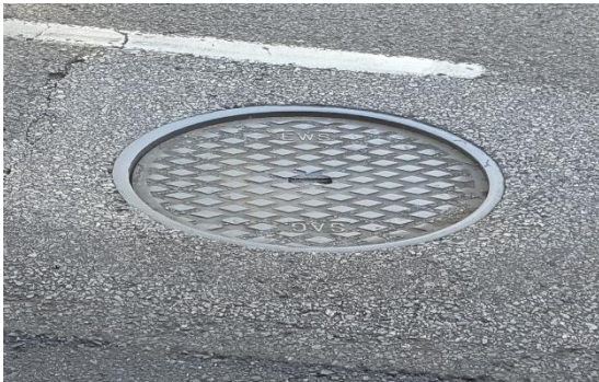
Many sewer plates are sunken in the housing
