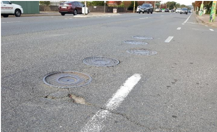
Series of 5 covers at the intersection with Andrew Avenue
